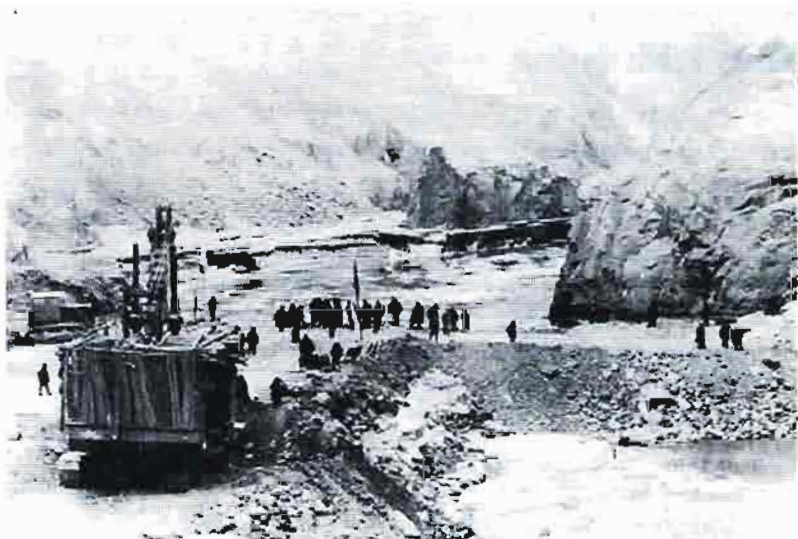
Construction of the Longyang Gorge Hydropower Station is under way. Damming of the river has been completed.
