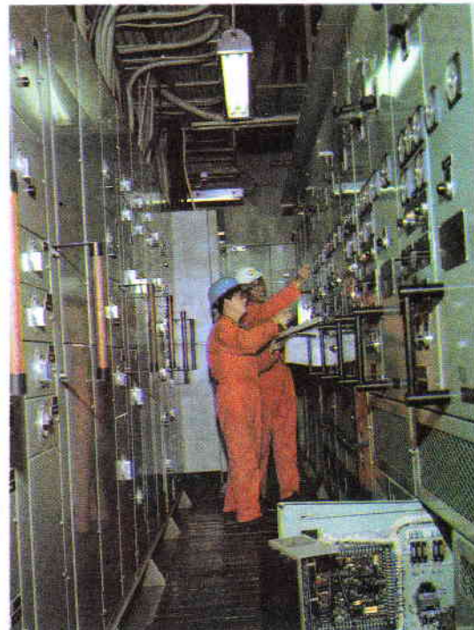
The platform's power center.
