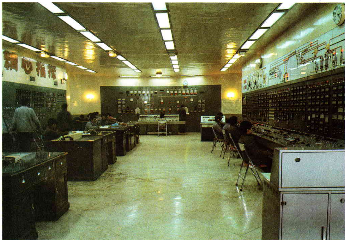
The control center at Yaomeng power plant's No. 1 generating unit. Li Fen
