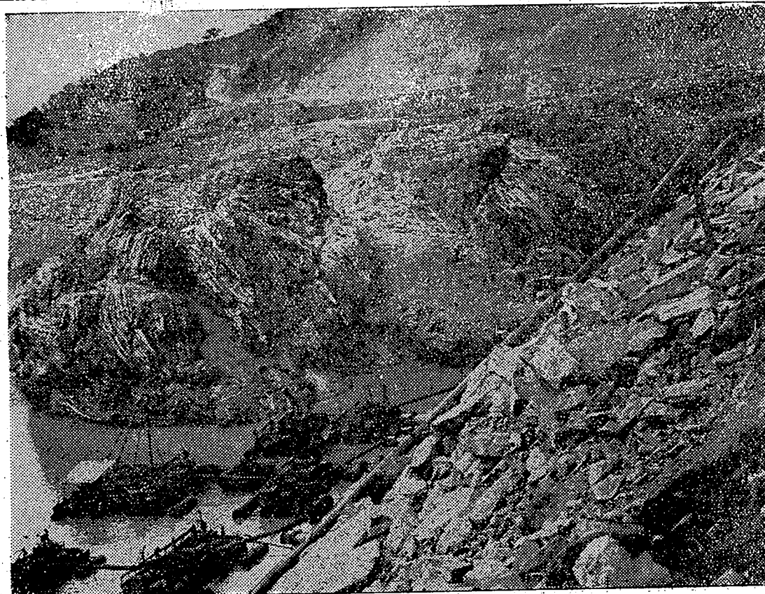
Prototype dredgers used for pumping out water trapped between the two coffer-dams. 27 such pumps were used in the watering programme which lasted just under 3 weeks.
